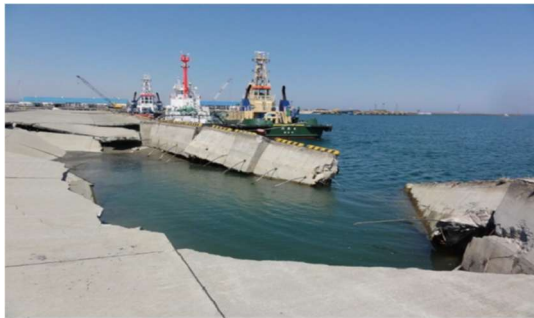
Figure 6 Damage to a Steel Sheet Pile Quay Wall at Soma Port During the 2011 Tohoku Earthquake Off the Pacific Coast (Sugano et al., 2014)
