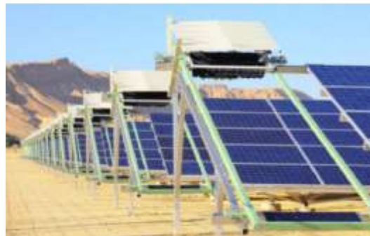
(b) Automated facility for cleaning
